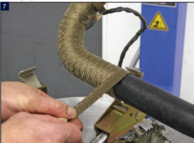
7 The key word here is "tight". Every pass that you make around the pipe, be sure to pull the wrap very tightly.
